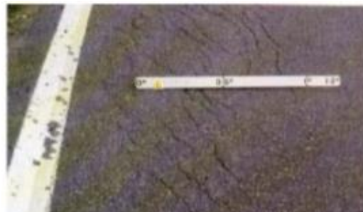
Gambar 3.34 Patah Slip ( Slippage Cracking )
