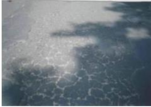
Gambar 3.38 Pelepasan Butir ( weathering and raveling )
