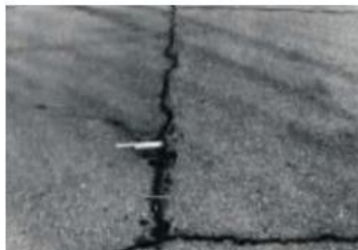
Gambar 3.16 Retak Sambung ( Joint Reflec Cracking )
