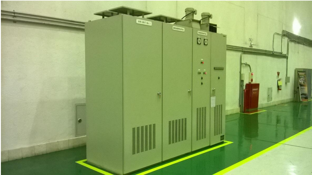
Gambar 4.6 Panel AVR, Surge Absorber , dan Thyristor di PLTA Musi
