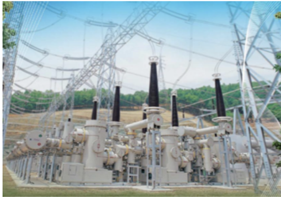
Gambar 2.4 Gas Insulated Substation (GIS)
