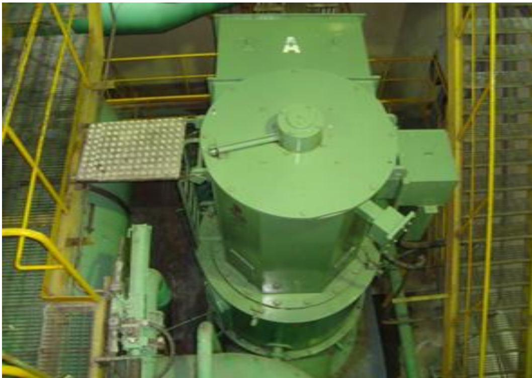
Gambar 2.10 Main Cooling Water Pump
