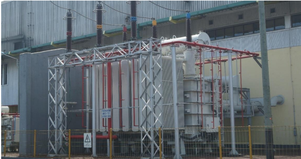
Gambar 2.13 Main Transformator 11.8 KV /150 KV
