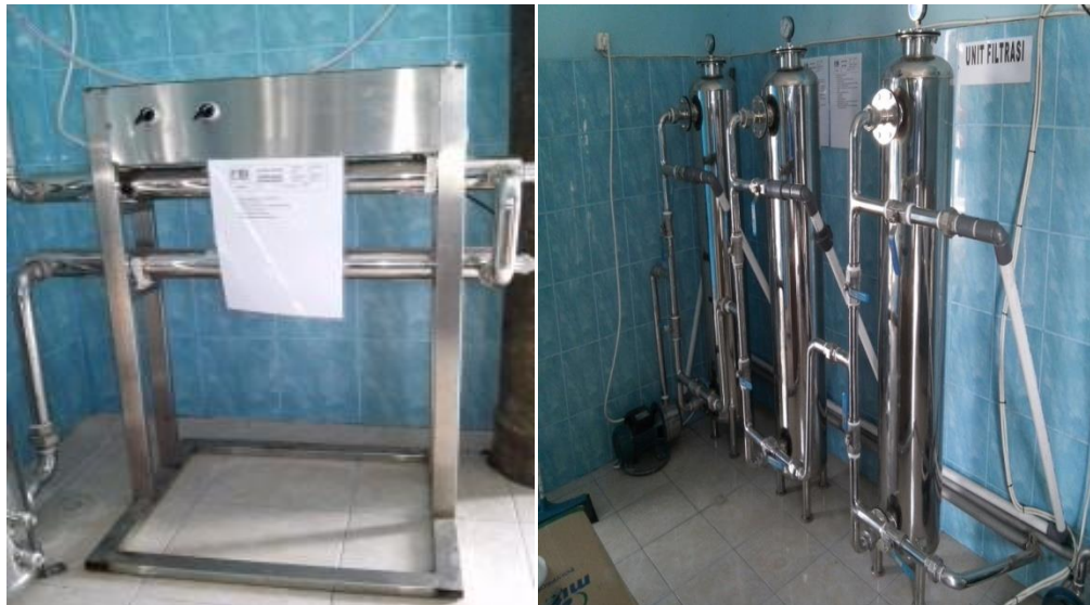
Gambar Unit Mesin Pengolahan Air ( Water Treatment )
