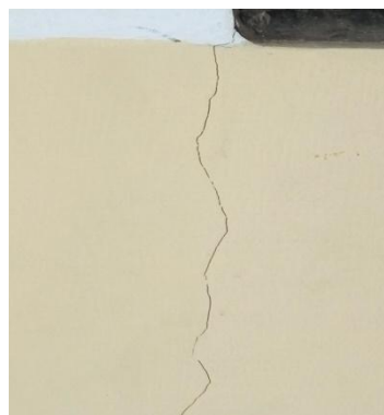
Gambar 5.47 Dinding retak diagonal SD N Gungan
