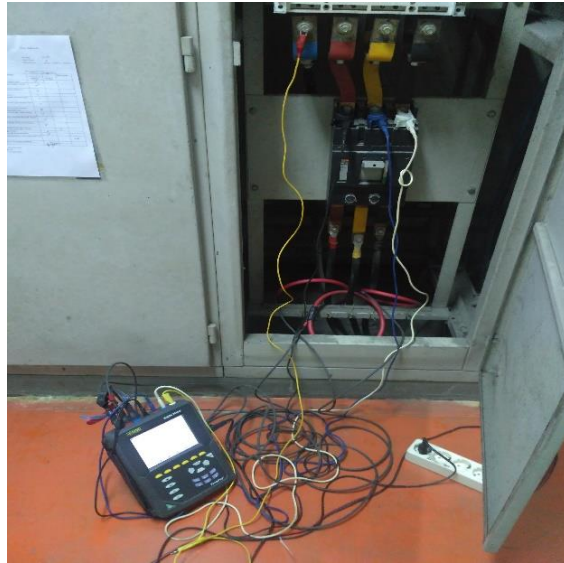
Gambar 3.2 Instalasi Power Analyzer
