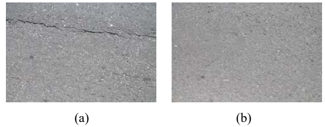
Figure 8. Middle quality images (a) crack, (b) non-crack
