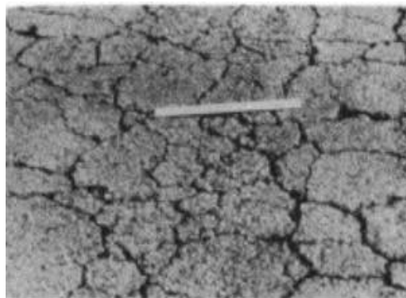
Gambar 2.5 Retak Kulit Buaya ( Aligator Cracking ) Sumber : Bina marga no.03/MN/B/1983
