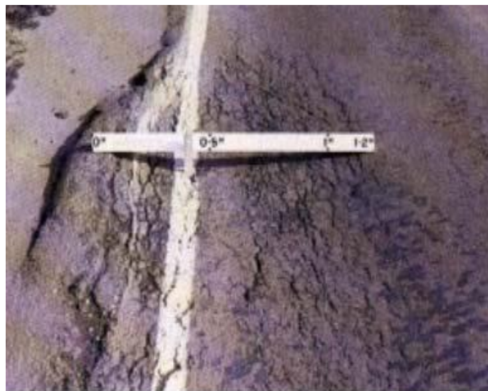
Gambar 2.34 Sungkur ( Shoving ) Sumber : Bina marga no.03/MN/B/1983
