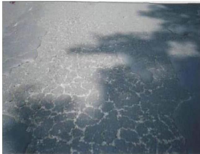
Gambar 2.40 Pelepasan Butir ( Weathering/Raveling ) Sumber : Bina marga no.03/MN/B/1983
