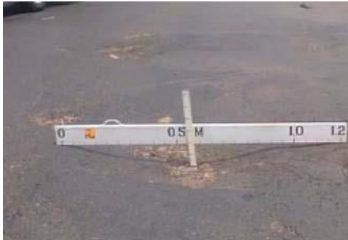
Gambar 2.15 Amblas ( Depression ) Sumber : Bina marga no.03/MN/B/1983
