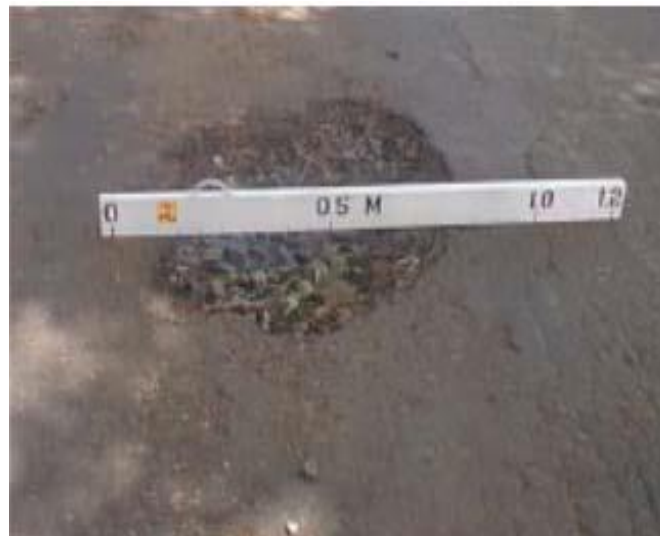
Gambar 2.28 Lubang ( Pothole ) Sumber : Bina marga no.03/MN/B/1983
