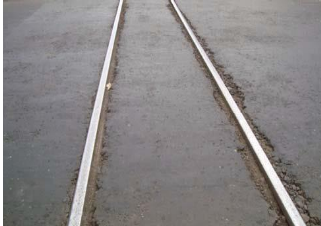
Gambar 2.30 Rusak Perpotongan Rel ( Railroad Crossing ) Sumber : Bina marga no.03/MN/B/1983
