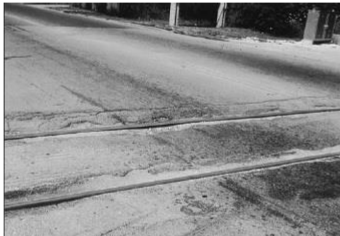
Gambar 3.27 Rusak Perpotongan Rel ( Railroad Crossing )
