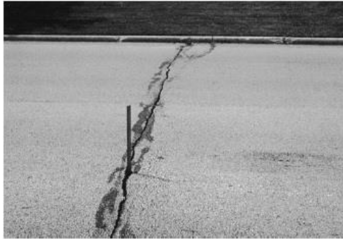
Gambar 3.19 Retak Memanjang/Melintang ( Longitudinal and Transverse Cracking )
