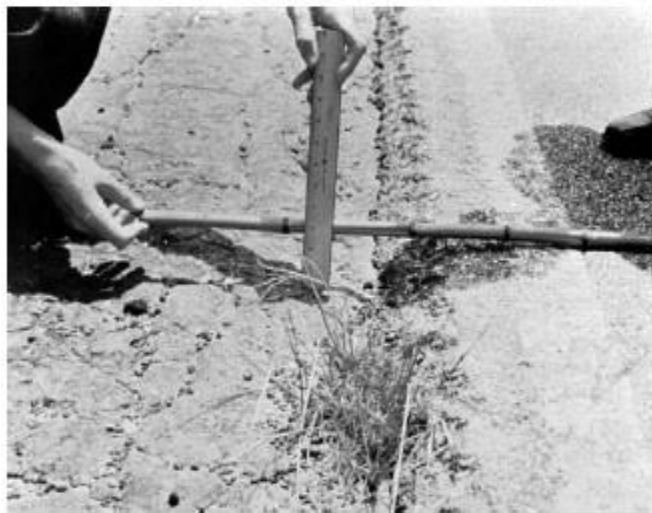
Gambar 3.17 Pinggir Jalan Turun Vertikal ( Line/Shoulder Dropp Off )
