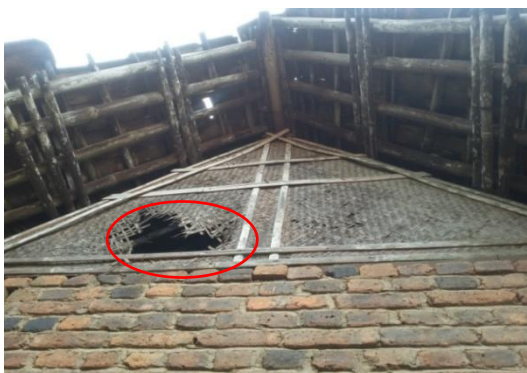
Gambar 4.27 Exterior Falling Hazard ( Sumber : Survei Lapangan 2018 )
