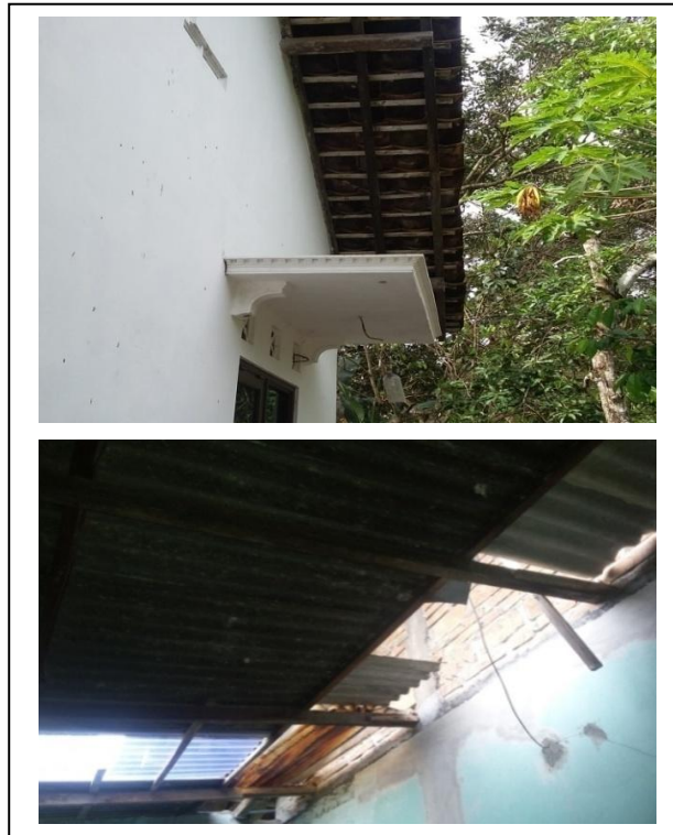
Gambar 4.6 Exterior Falling Hazard ( Sumber : Survei Lapangan 2018 )
