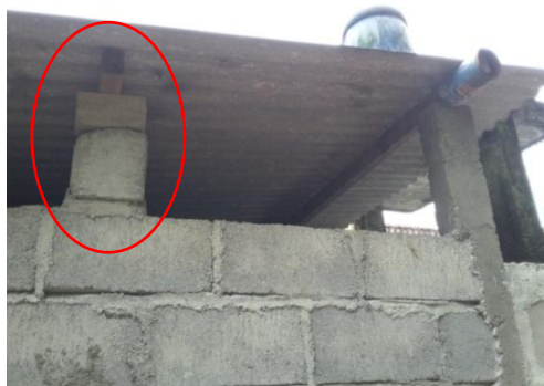
Gambar 4.37 Exterior Falling Hazard ( Sumber : Survei Lapangan 2018 )
