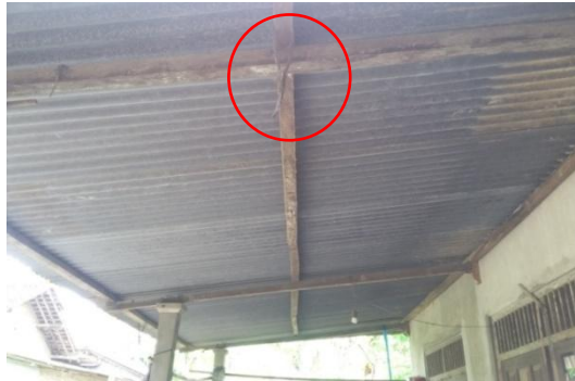
Gambar 4.15 Exterior Falling Hazard ( Sumber : Survei Lapangan 2018 )
