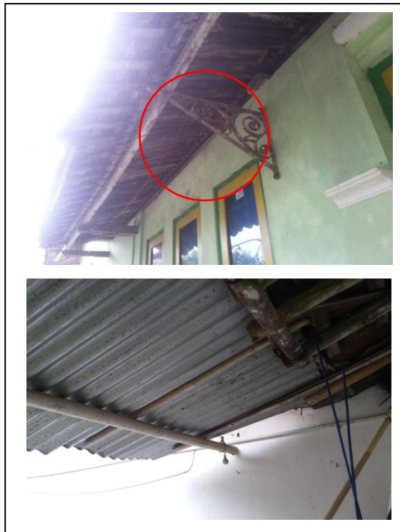
Gambar 4.53 Exterior Falling Hazard ( Sumber : Survei Lapangan 2018 )
