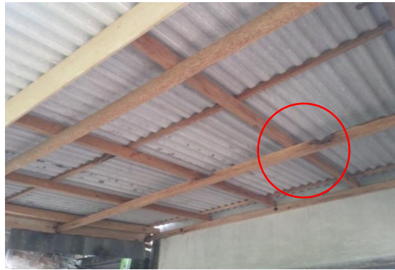
Gambar 4.20 Exterior Falling Hazard ( Sumber : Survei Lapangan 2018 )
