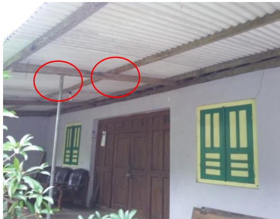
Gambar 4.42 Exterior Falling Hazard ( Sumber : Survei Lapangan 2018 )
