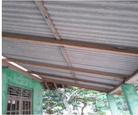
Gambar 4.10 Exterior Falling Hazard ( Sumber : Survei Lapangan 2018 )
