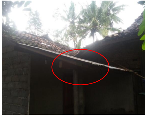
Gambar 4.32 Exterior Falling Hazard ( Sumber : Survei Lapangan 2018 )
