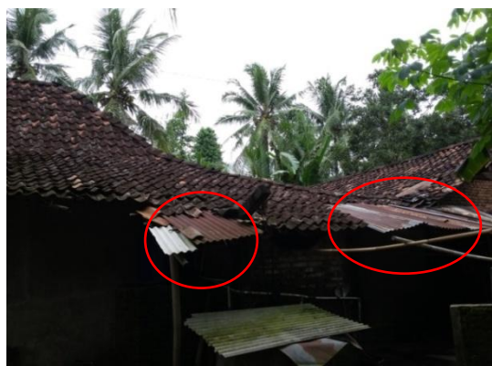
Gambar 4.47 Exterior Falling Hazard ( Sumber : Survei Lapangan 2018 )
