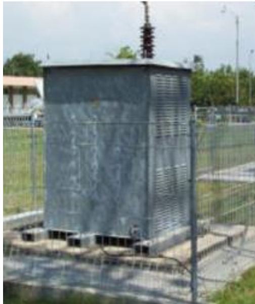
Gambar 2.20 NGR ( Neutral Grounding Resistor )
