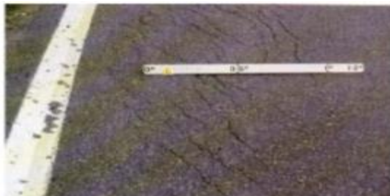
Gambar 2.37 Patah Slip ( Slippage Cracking )
