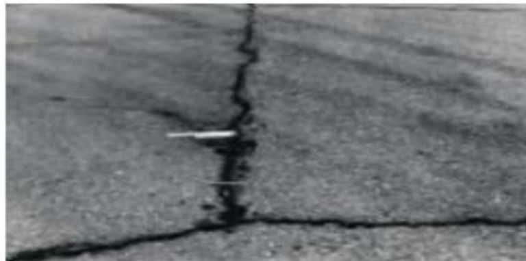
Gambar 2.19 Retak Sambung ( Lane Joint Cracks )
