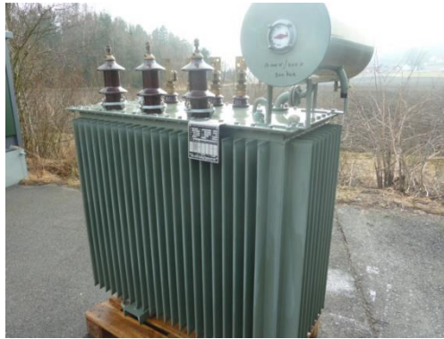
Gambar 2.5 Transformator distribusi step down 500 kVA
