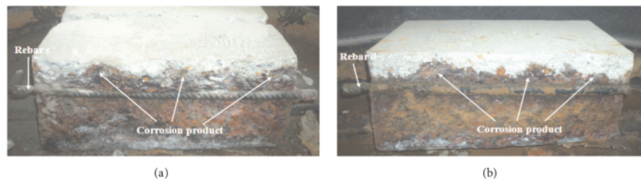
FIGURE 16: Cut sections of the postcorrosion slab: (a) rebar c and (b) rebar d.
