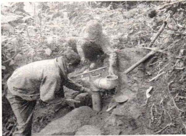
Picture 4) The villagers plant hydram pipe to bring up water level from the water source. With this technique, the villagers can obtain clean water. Before, the villagers had to walk for around 2 km down the hill to get the clean water
