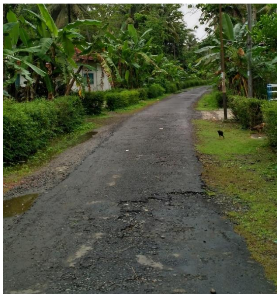
Picture 3.3 Village Road Condition of Pringgowijayan Village
