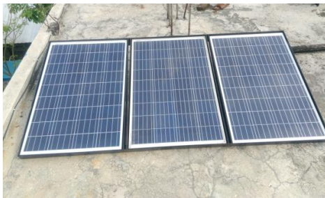
Gambar 4.4 : Panel surya Solar Home System MBS
