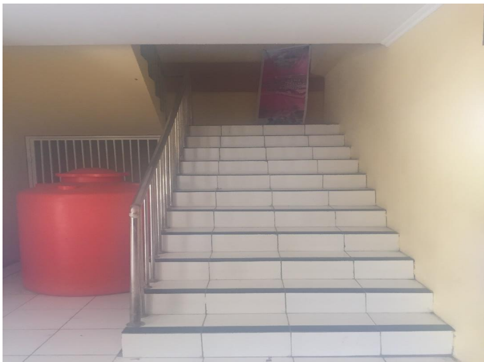
Figure 3.7 Condition of stairs at SMAN 4 Kota Palu
