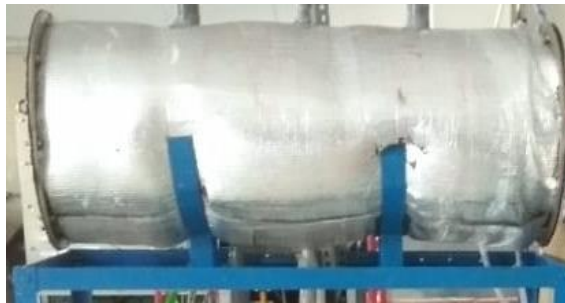
Gambar 3.4 Tangki Solar Water Heater
