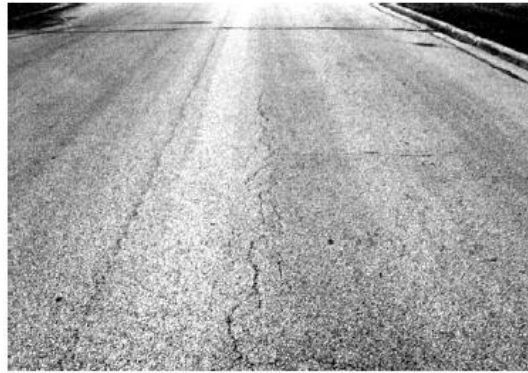
FIG. X1.1 Low-Severity Alligator Cracking
