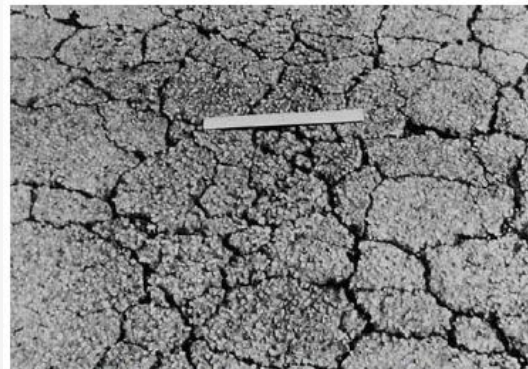
FIG. X1.3 High-Severity Alligator Cracking
