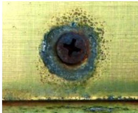
Gambar 2.2 Korosi galvanis (Mechanicalengineering, 2014)
