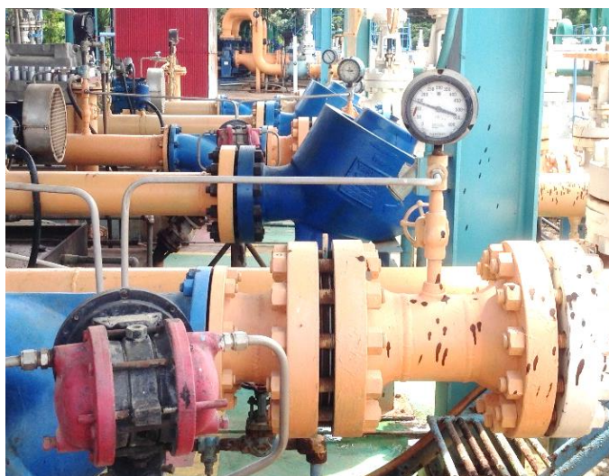
Gambar 3.3. Suction pressure gauge pompa injeksi
