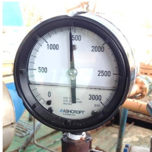
Gambar 3.4. Discharge pressure gauge pompa injeksi
