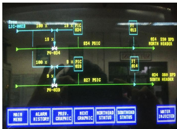
Gambar 3.2. Layar kontrol PLC Water Injection Plant (WIP)
