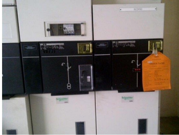
Gambar 2.2. Kubikal Tegangan Menengah Merk Schneider Electric (Sumber: http://www.indotrading.com/product/p24935.aspx )
