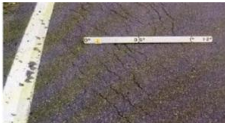
Gambar 3. 35. Patah Slip ( Slippage Cracking )
