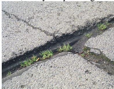
Gambar 3.16 Retak Sambung ( Joint Reflec Cracking ) Sumber : Bina Marga No.03/MN/B/1983
