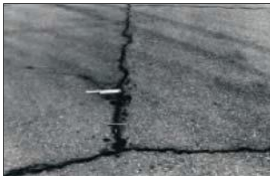
Gambar 3.16 Retak Sambung ( Joint Reflec Cracking )
