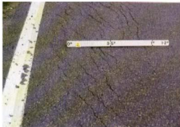
Gambar 3.34 Patah Slip ( Slippage Cracking )
