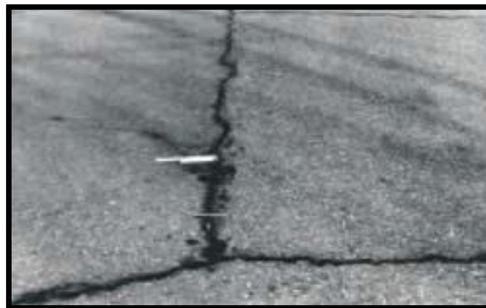
Gambar 3.17 Retak Sambung ( Joint Reflec Cracking )
