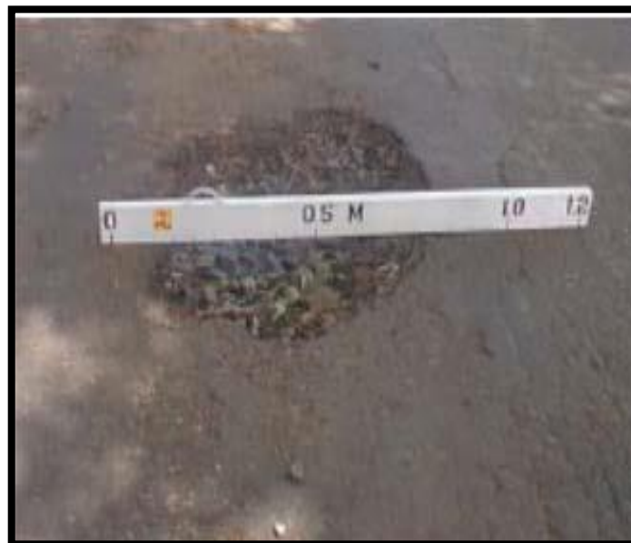
Gambar 3.27 Lubang ( Pothole ) Sumber : Bina marga no.03/MN/B/1983
