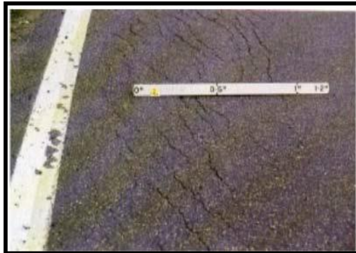
Gambar 3.35 Patah Slip ( Slippage Cracking )
