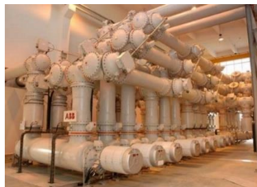
Gambar 2.3 Gas Insulated Substation
