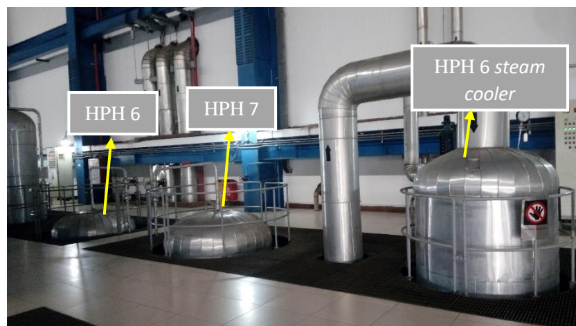
Gambar 2.19 High Pressure Heater PLTU Indramayu (Sumber: PLTU Indramayu)
