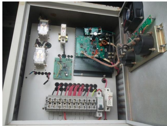
Gambar 2.5 Box Kontrol Turbin Angin
