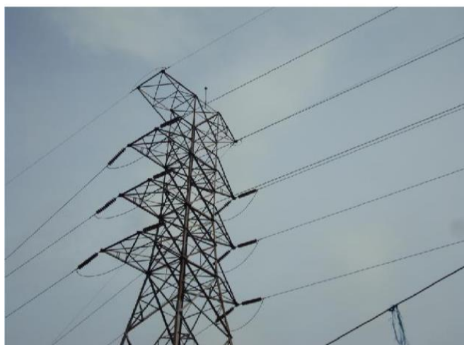
Gambar 2.19. Tower SUTT 150 KV jenis aspan/tension
