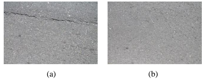
Figure 8. Middle quality images (a) crack, (b) non-crack
