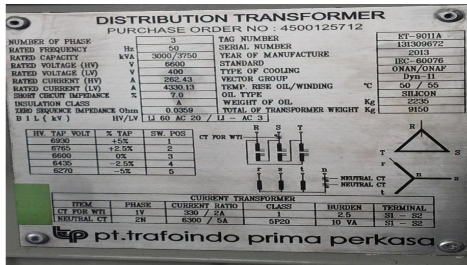
Gambar 2.18. Name Plate Transformator
