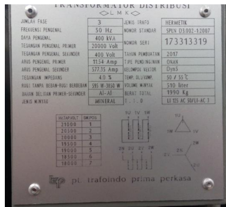
Gambar. 3.1. Data name plate transformator
