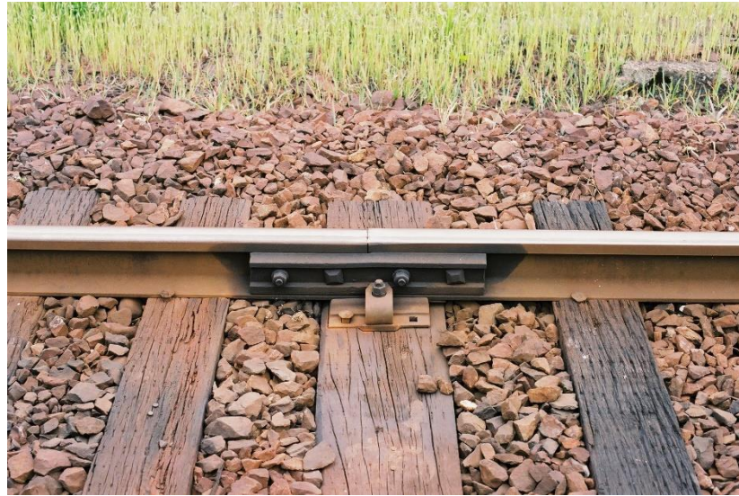
Gambar 3.6 Conventional Jointed Rails
